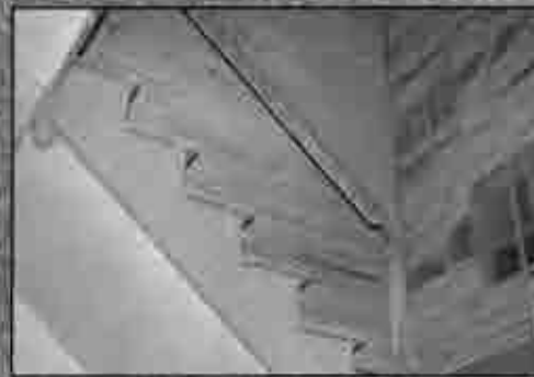
A staircase in its current condition in the Octagon House
